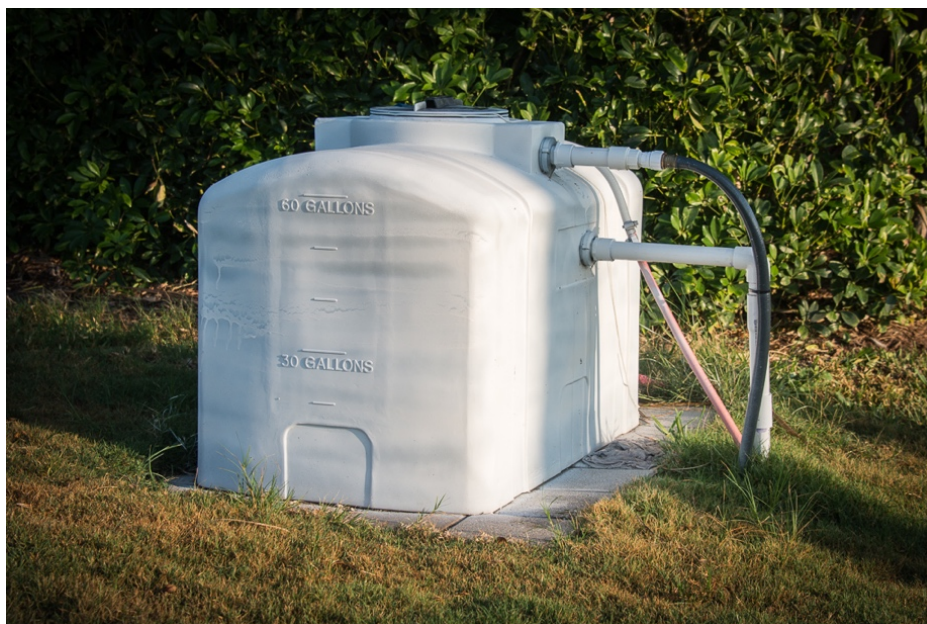
This is a TRM Biologics, self- contained Bio-Zyme Bio-Generator System.
